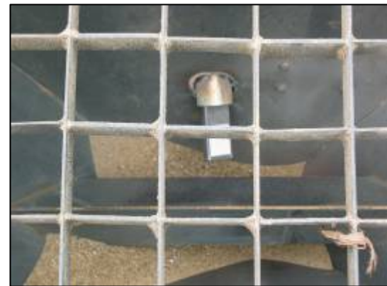
4 Ensure a good flow of material. Here a mesh is fitted for sensor protection
